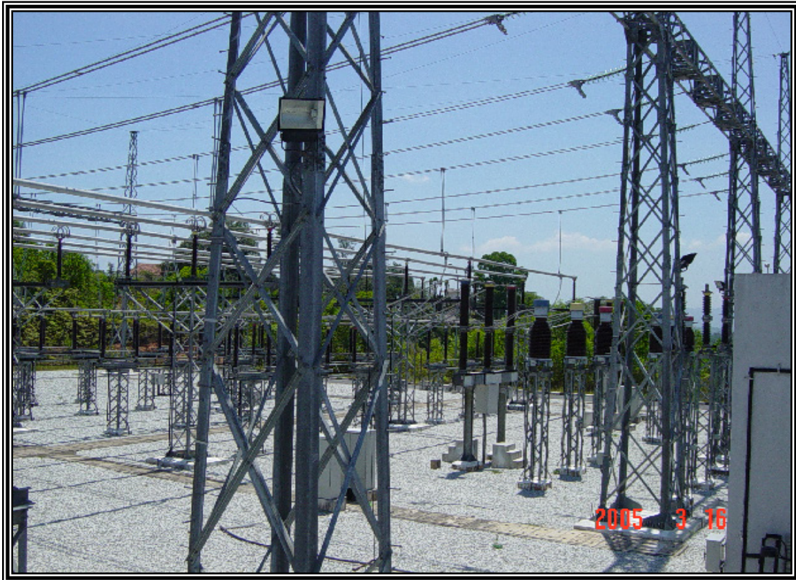
132/33/11kV Pasir Panjang Substation
