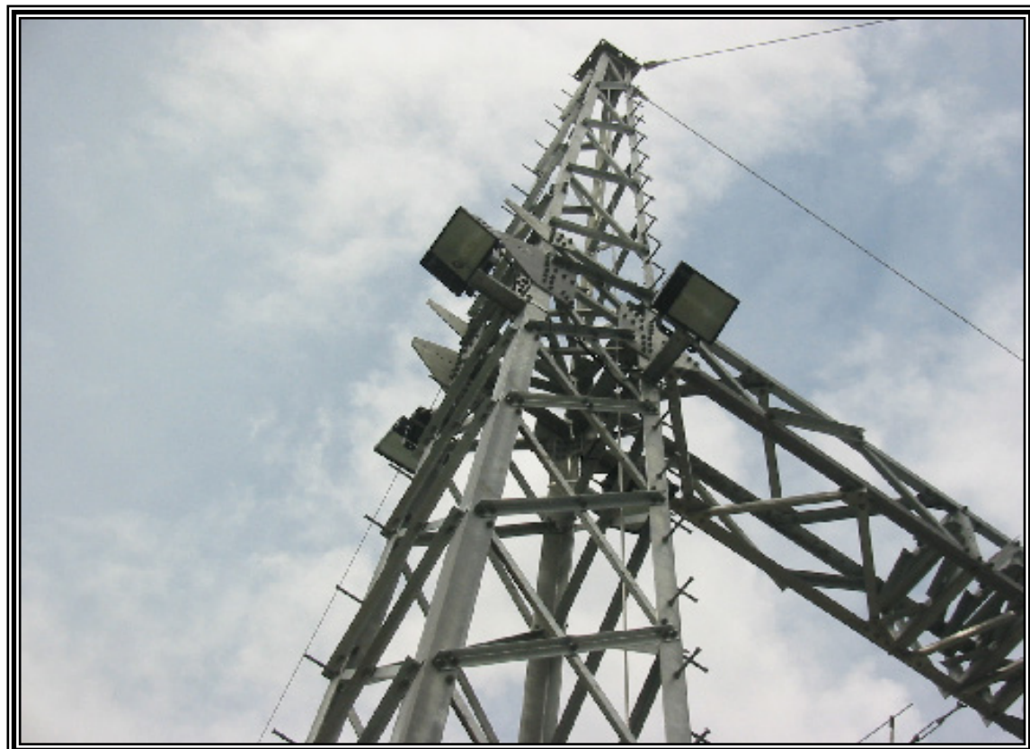
275kV Tg. Bin Substation
